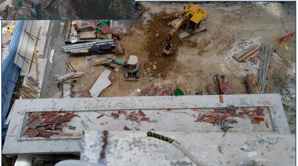
Guard Room, Water Meter Room & Ball Court Area – Preparation works for construction of ball court in progress.
