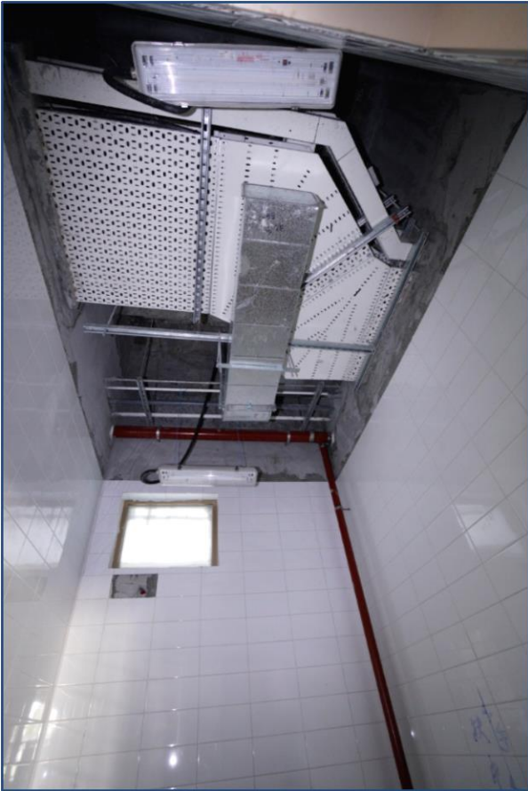
G/F Store Room next to Hub Room
