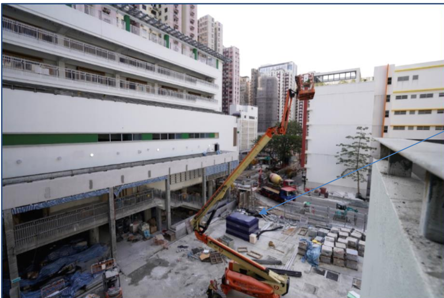
Chiller for Assembly Hall delivered to Site
