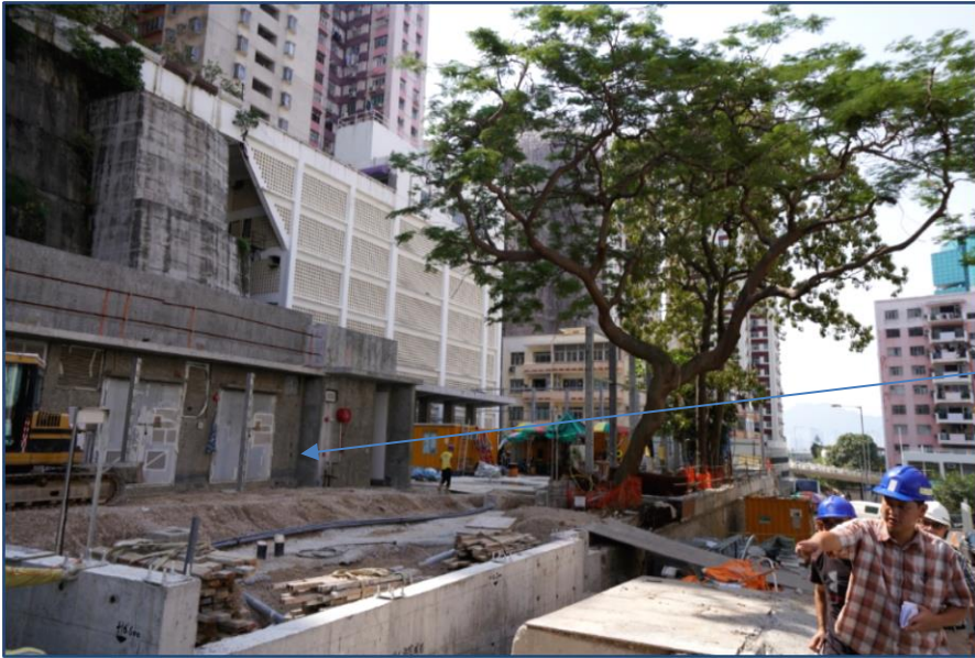
Transformer Room and Ball Court Area
