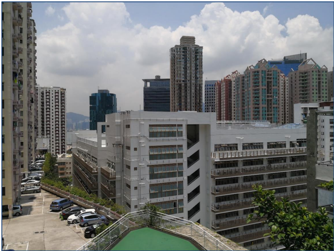
Installation of air-conditioners in progress. Installation of false ceiling support grids in progress.
